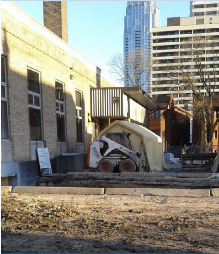
The Postal Station K's rear-end being demolished, image by UrbanToronto Forum contributor Roundabout
